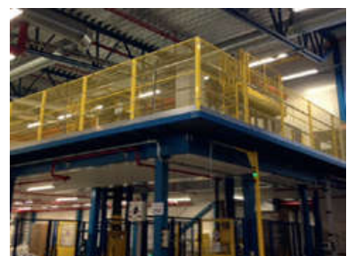
12 Mezzanine Guard Fall protection on Mezzanine floor areas.
